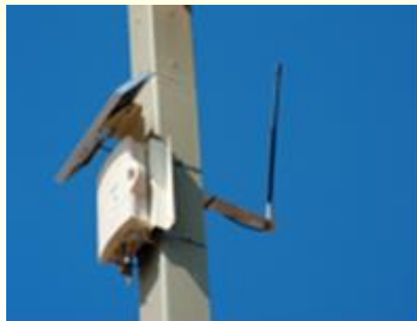
Solar-powered wireless relay for AMR
