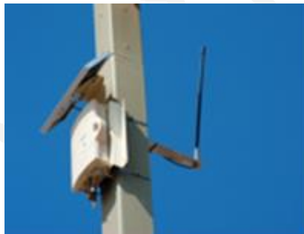
Solar-powered wireless relay for AMR
