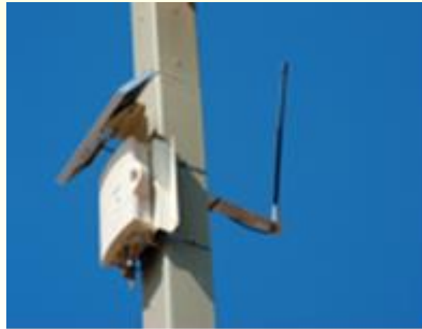
Solar-powered wireless relay for AMR
